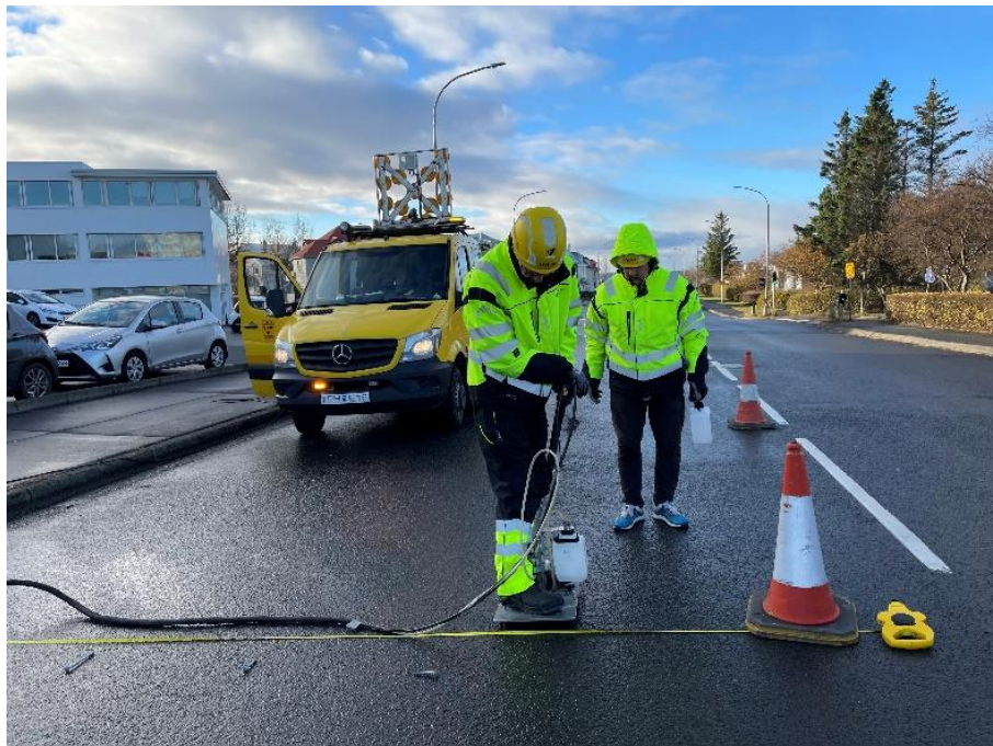
Figure 136. WDS measurements at Hofsvallagata on 20 October 2022.
